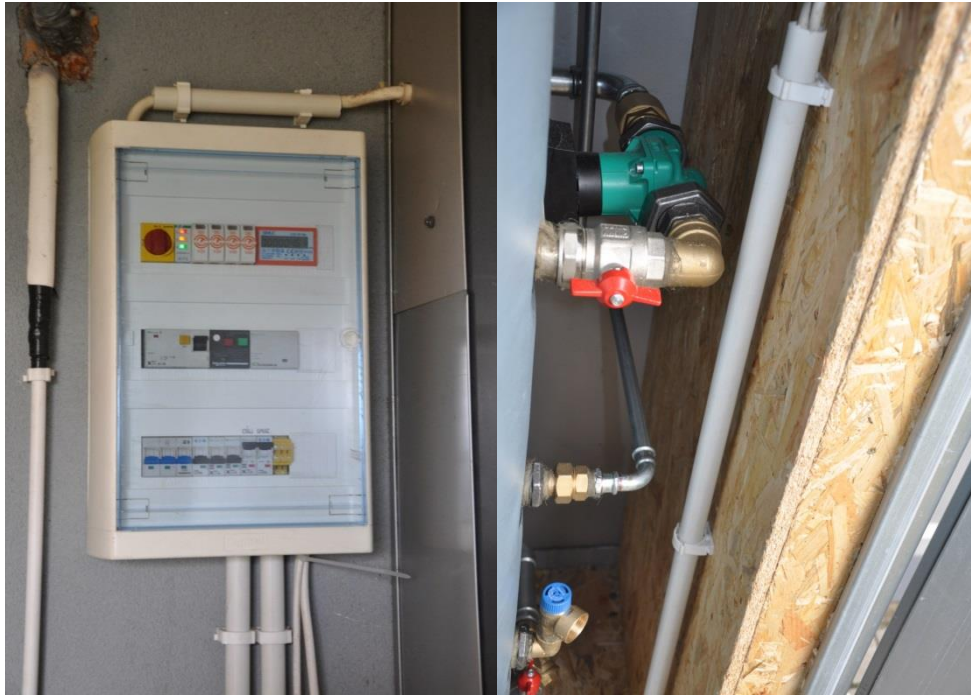
Figure 6-6. Pilot installation of heat pump in Armada Development
