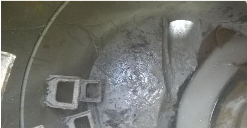
Figure 6-4. CZOK drain with mine water (to be connected with buffer tank)
