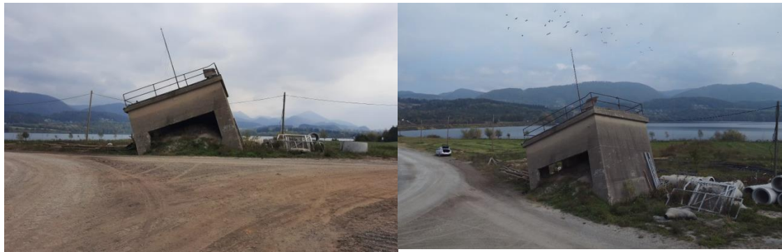
Figure 2-4. Example of subsidence of the surface caused by lignite excavation in Premogovnik Velenje coal mine
